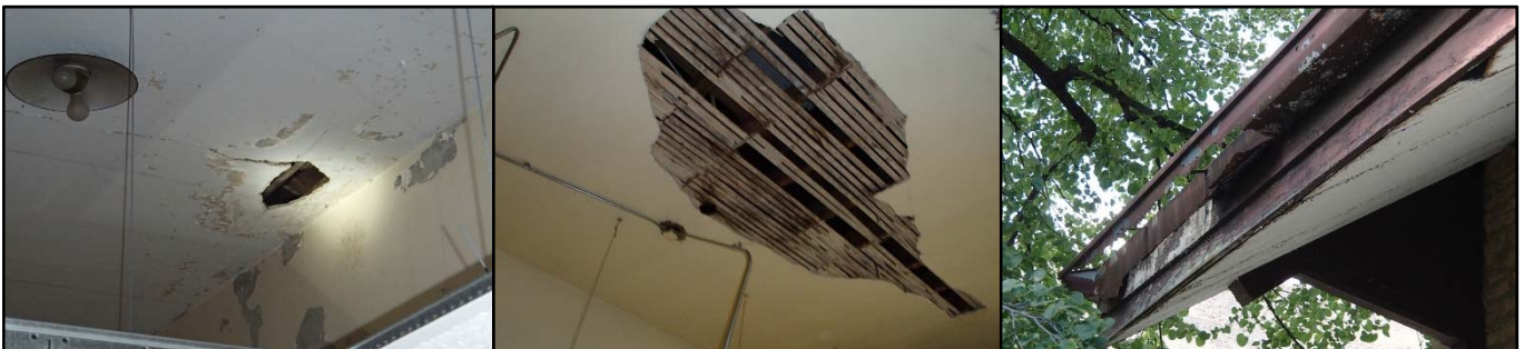
SHAPIRO DEVELOPMENT CENTER ENGINEERING BUILDING DAMAGE
