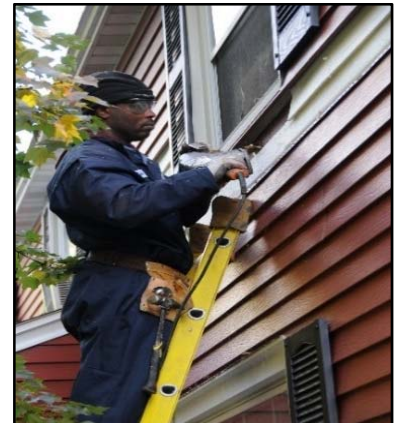
UPDATING WINDOW INSULATION WILL REDUCE ENERGY COSTS
