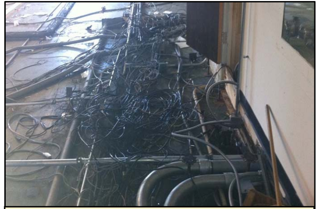
REMAINING CORDS OF A SERVER ROOM IN THE ILLINOIS STATE ARMORY - SPRINGFIELD
